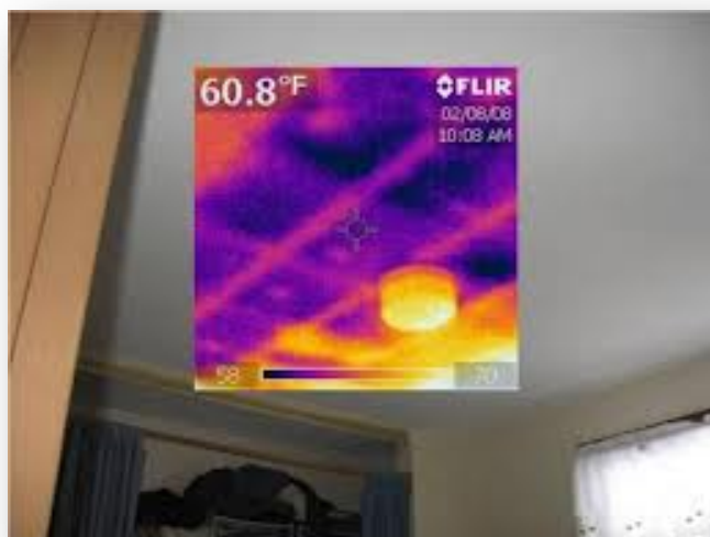
Booth Bay Register/Thermal imaging
