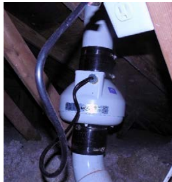
Radon Fan in Attic
