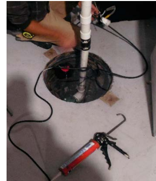
Radon Sump Pump Mitigation
