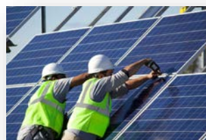
Solar PV installation
