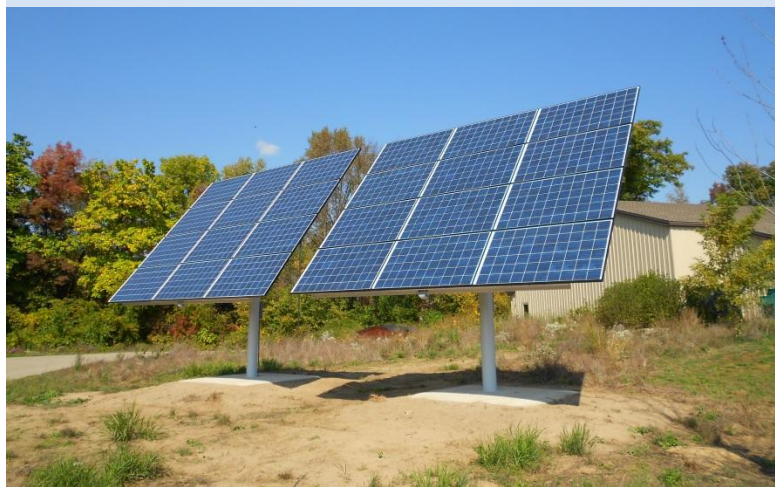
5.88kw solar panel array installed at the Gun Lake Tribe Community Center in Shelbyville, MI
